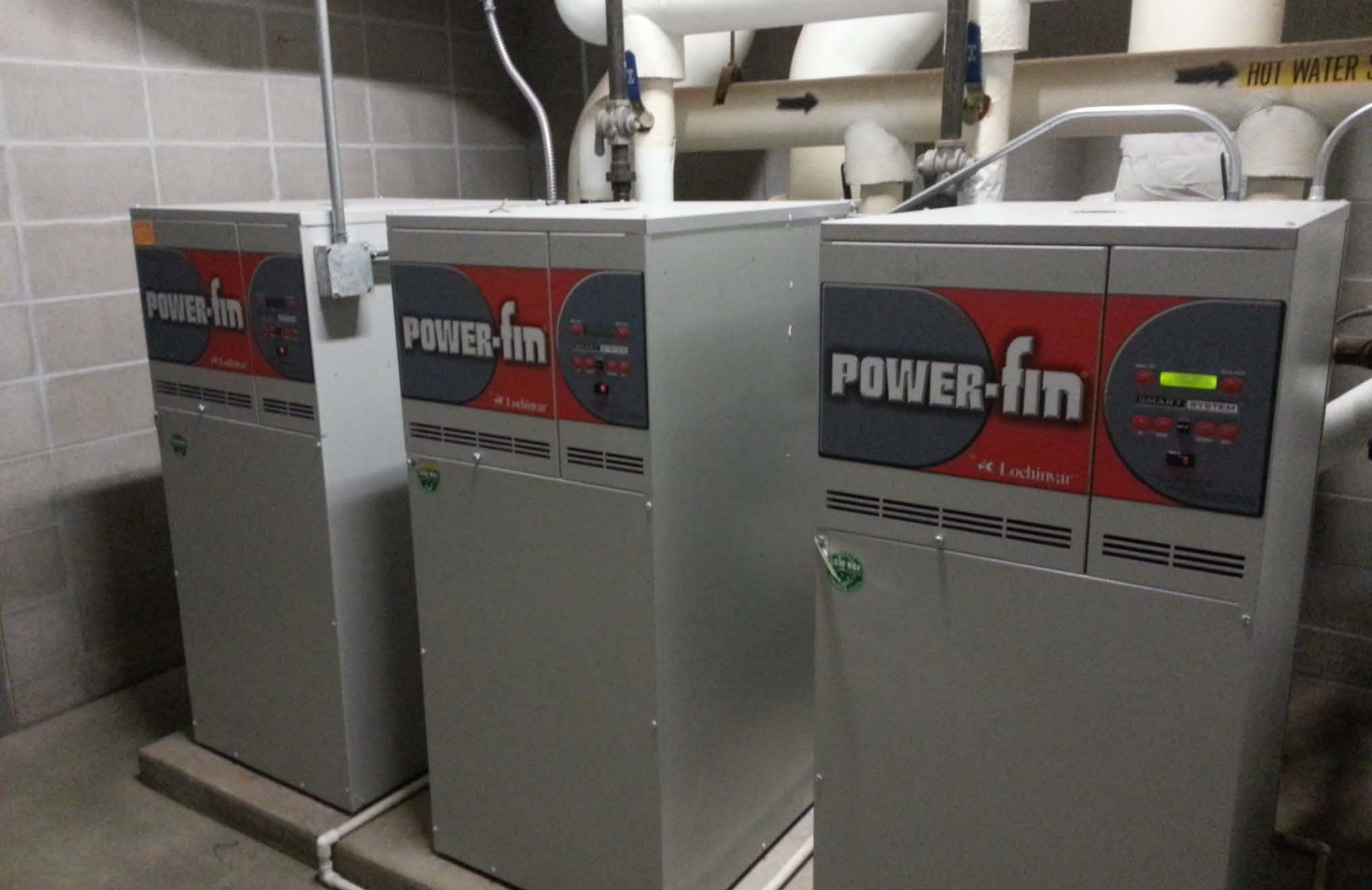
Boilers (Law Enforcement Center)
