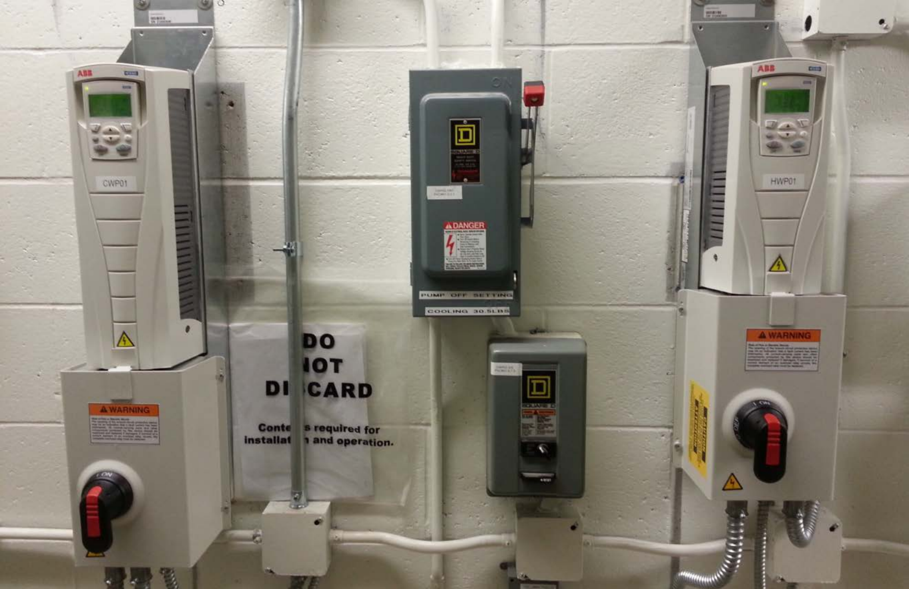
New Variable Frequency Drives (Annex)
